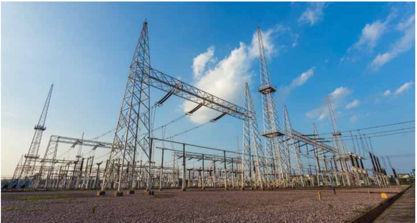
Switchyard Plant, Bhilai
