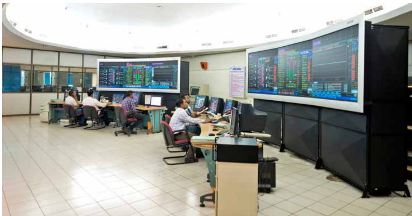
Bhilai PP-III Control Room
