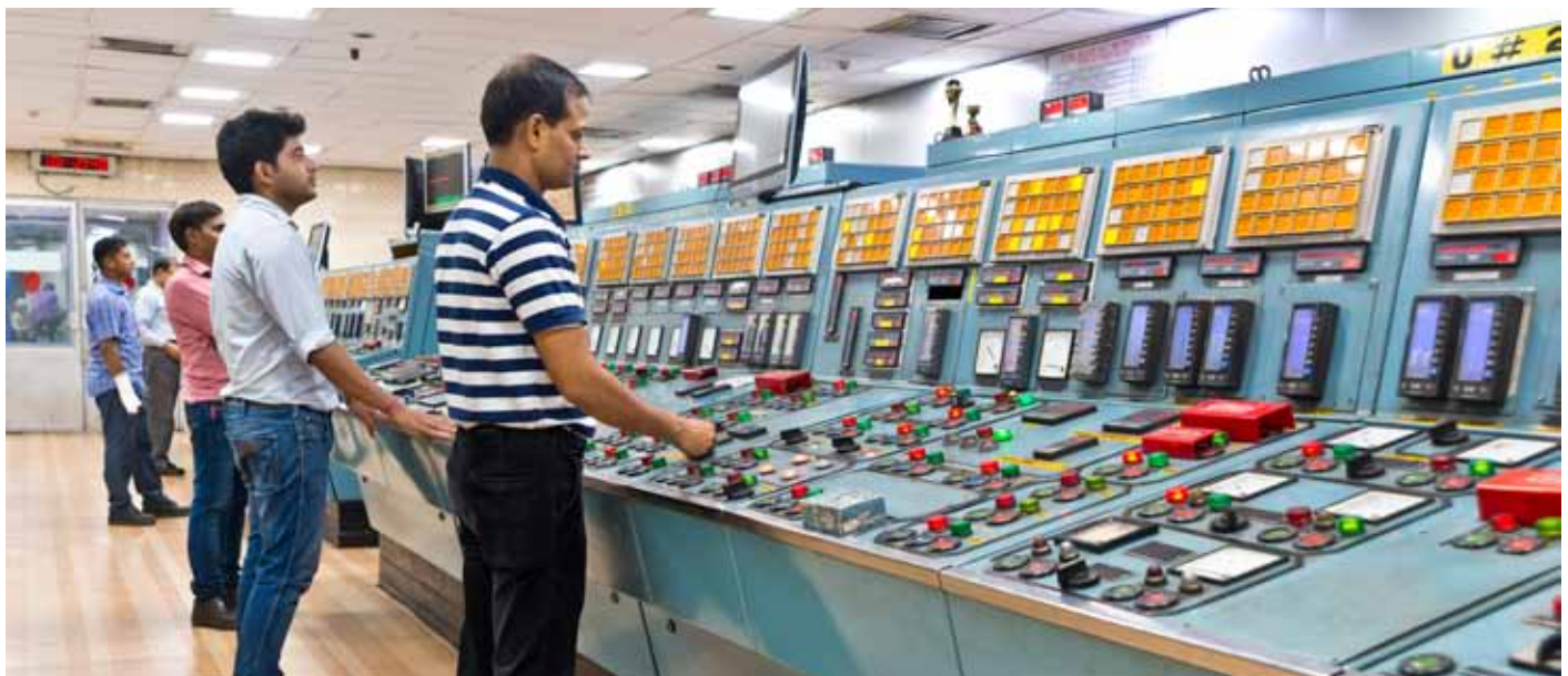
Durgapur Control Room
